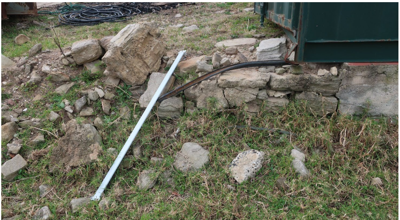
Photo 3-27 Remains of the rough stone cottage following a fire
